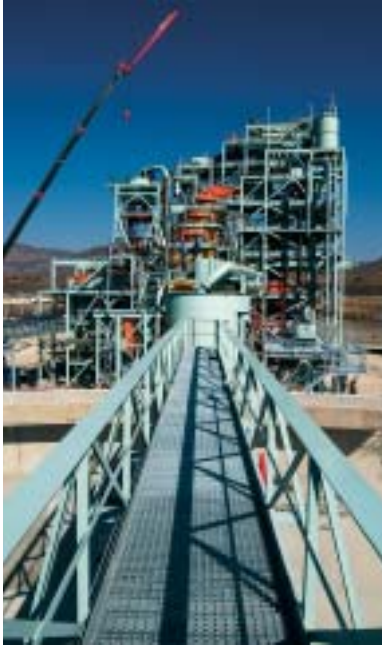
Construction of the concentrator at Impala Platinum's Marula operation on the eastern limb of the Bushveld Complex was completed in late 2003.
