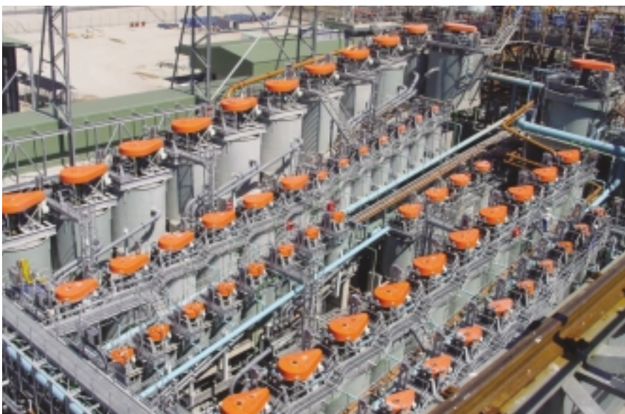
Flotation cells at the processing plant that serves Aquarius Platinum's Marikana mine. The plant was commissioned in November 2002.
